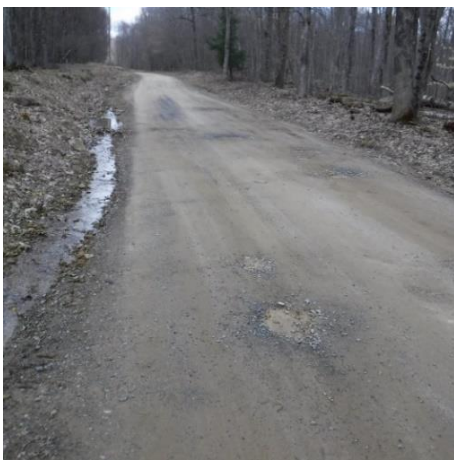
Saturated ditch and road base
