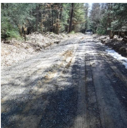
Saturated ditch and road base
