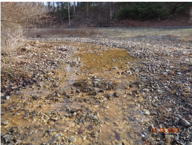
Standing water prior to maintenance
