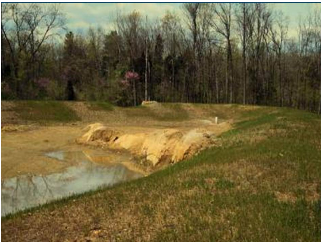
A leaking pond located in central Pennsylvania.
